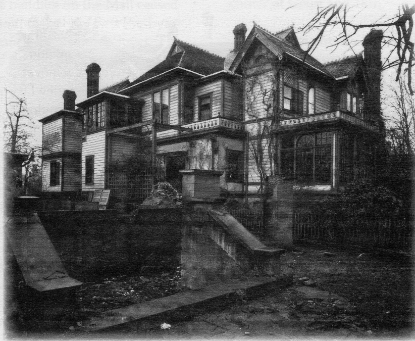
The A.N. Bush house just before demolition (courtesy of the Salem Public Library)
